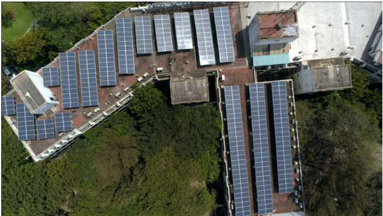
An Eagle eye view of the Rooftop Solar Power Plants installed at the Port's Administrative Office
