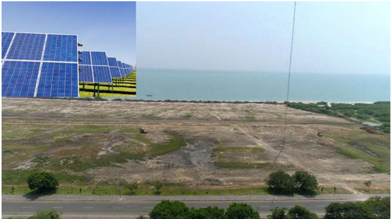
Work in progress for installing 5 MW Ground Based Solar Power plant at a cost of ₹25 Crore
