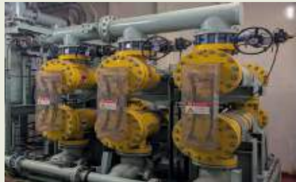
BWTS installed on SCI VLCC DESH VIRAT
