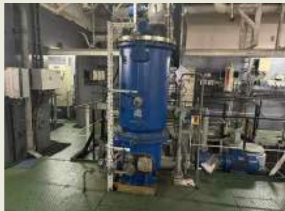
BWTS installed on SCI Container vessels SCI Chennai & SCI Mumbai
